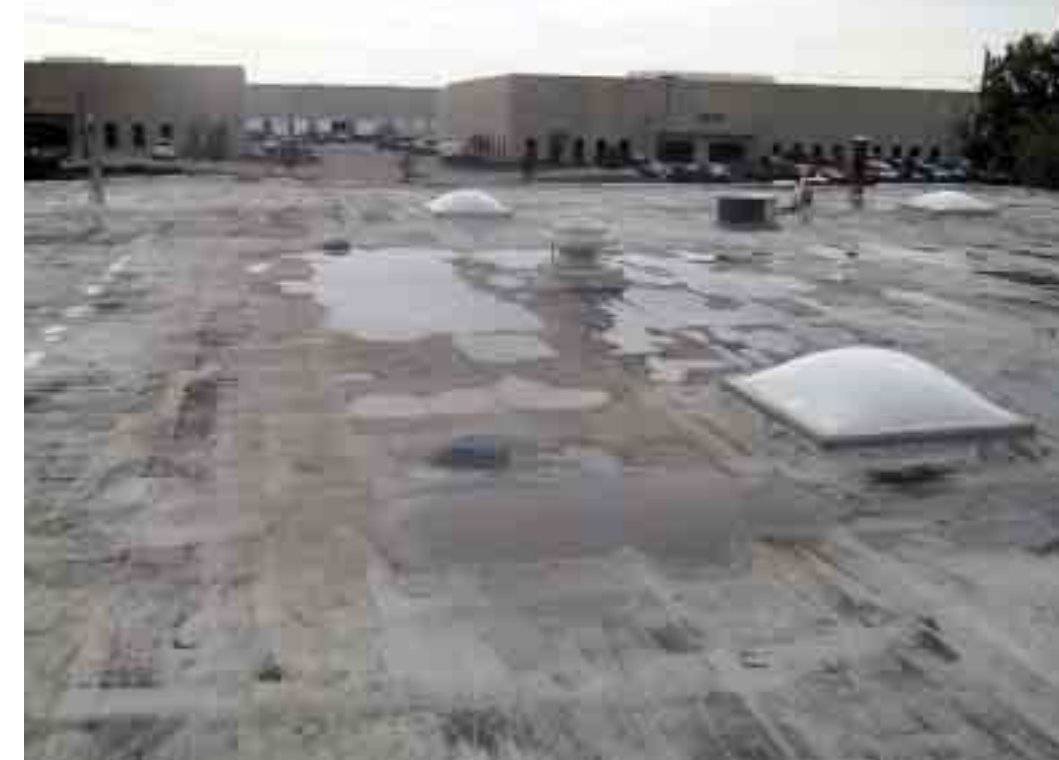
If moisture is accumulating anywhere in the building envelope, e.g. around doors, windows, in the roof, etc., aggressively look for the source of the leak and have it fixed quickly.
